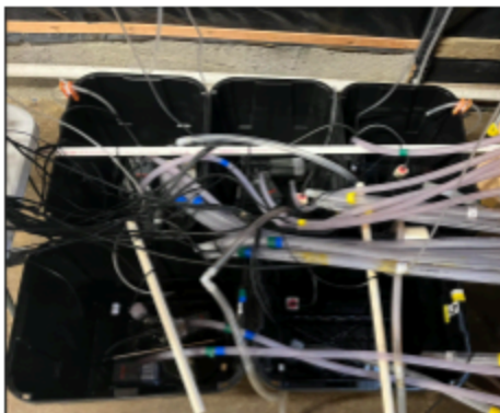
b. Temp. Controlled Reservoirs
